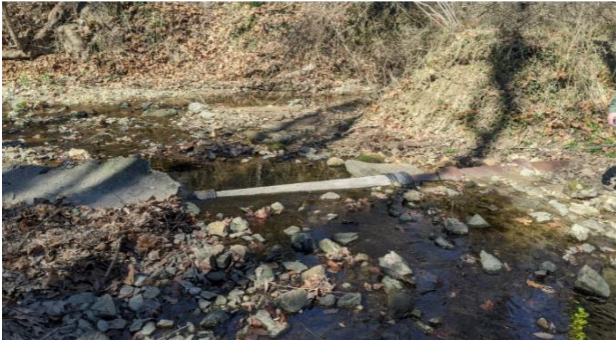
Figure 5: An exposed pipe, one of the at-risk WSSC sewer assets that will be addressed with Project
