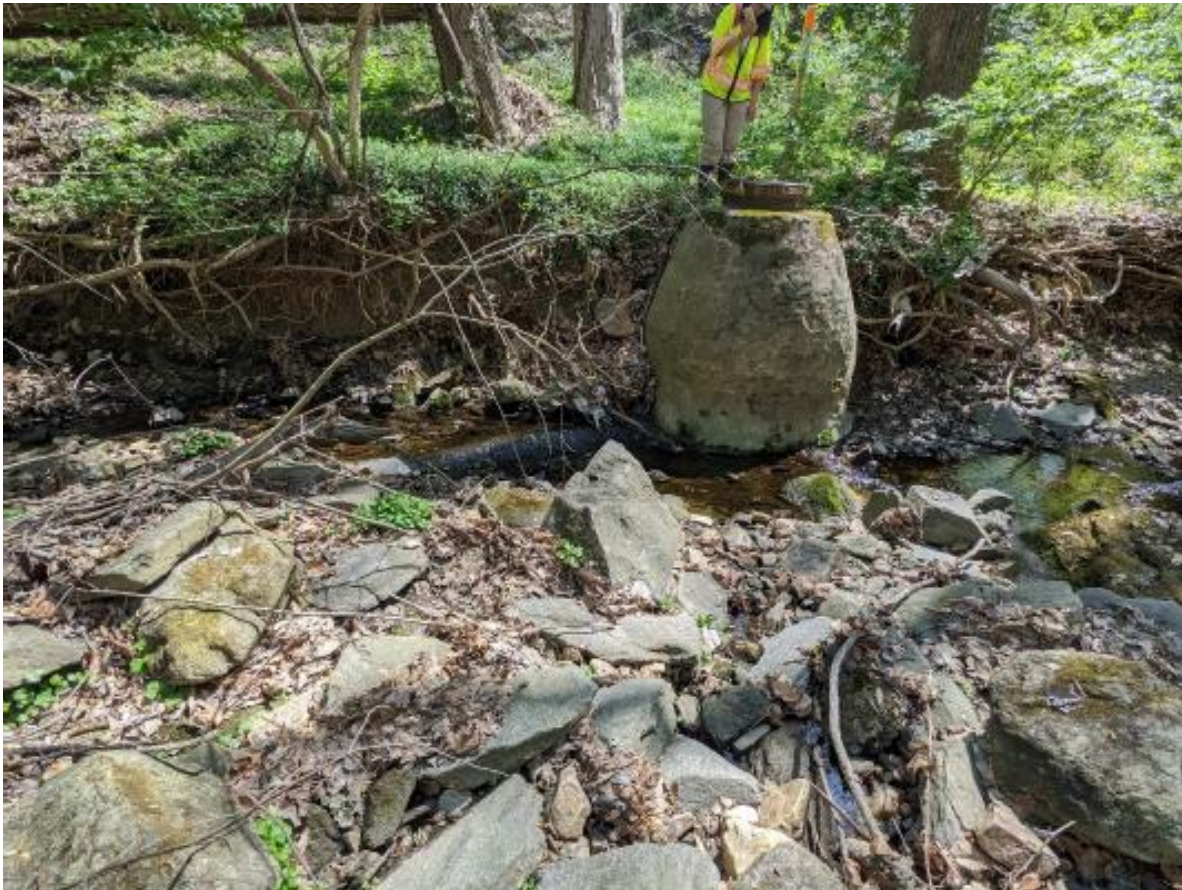
Figure 6: Exposed pipe and manhole, examples of at-risk WSSC sewer assets that will be addressed with Project
